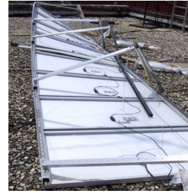
Fig. 4. Damage to a photovoltaic solar system caused by wind
